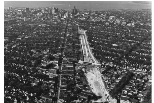
Figure 4. Construction of the Kensington Expressway, one of the major physical dividers of the East Side of Buffalo.
